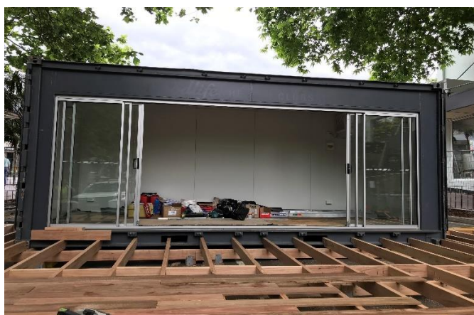
MAIN PAVILION - HIRED CONTAINER
