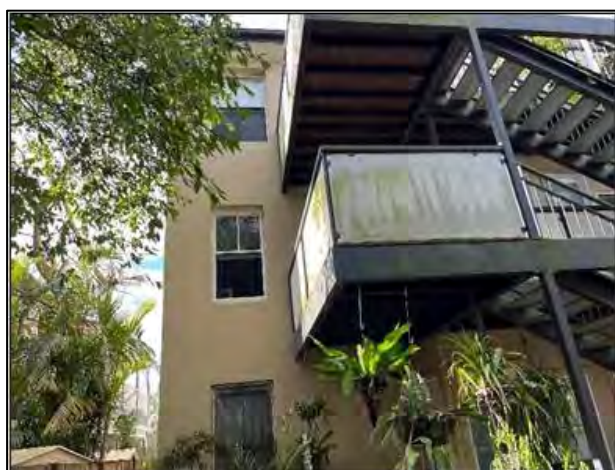
Figure 7. View of the north-wester corner of the building and the rear deck and stair structure.
