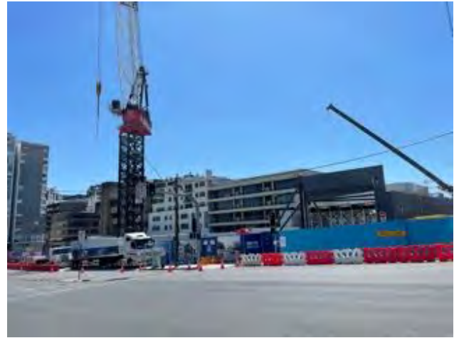
Picture 2 – Crows Nest Metro site to the north east of the site
