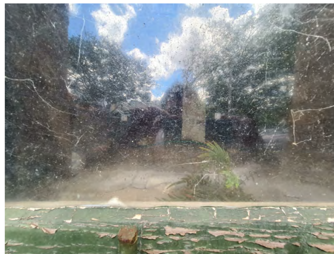
3 - EXISTING SUB-FLOOR SPACE (THROUGH NORTHERN HERITAGE WALL WINDOW) - EARTH AT SILL LEVEL
