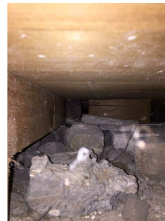
4 - EARTH UNDER FLOOR JOISTS OF GROUND FLOOR
