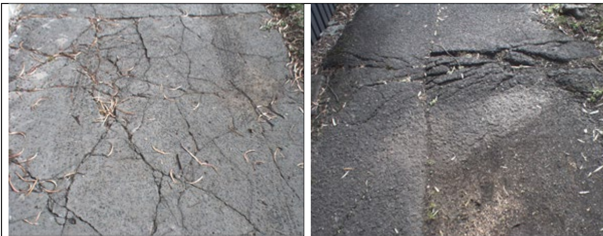
Asphaltic concrete footpath in poor condition
