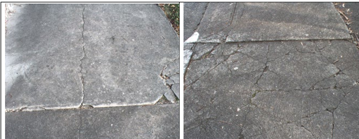
Concrete footpath in poor condition
