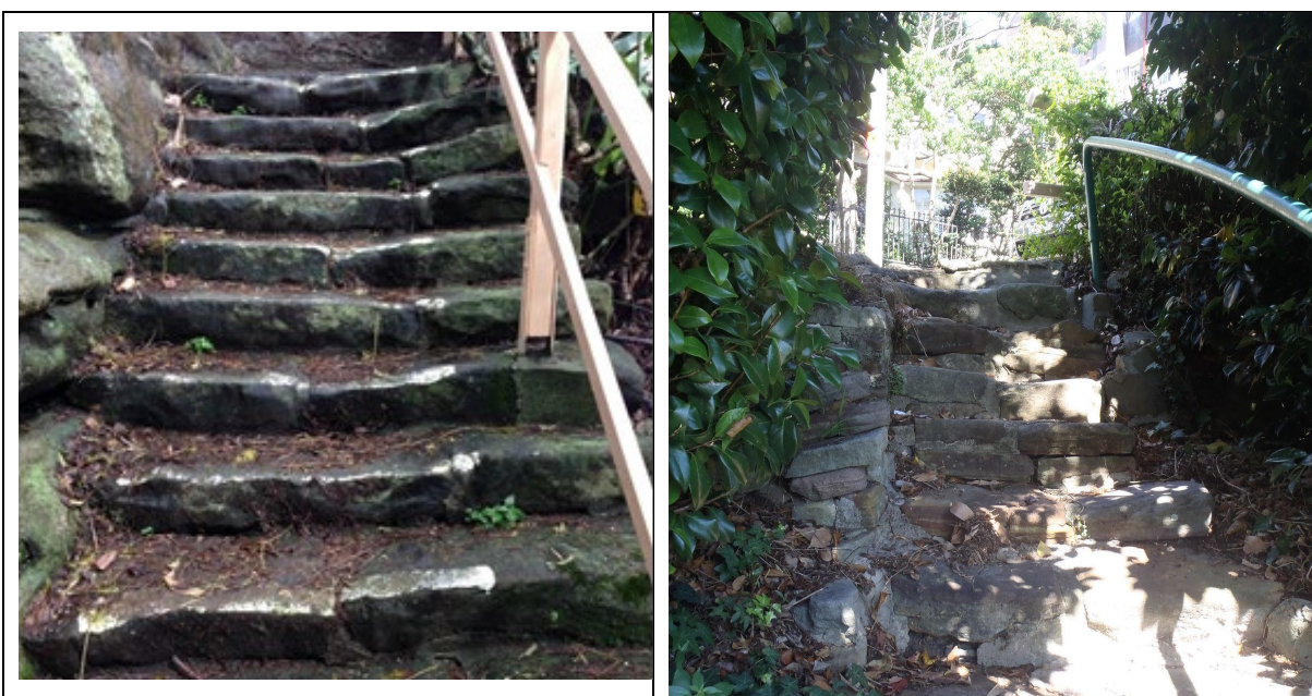
Stairs in poor condition
