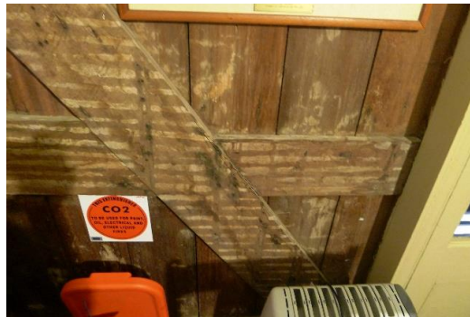
Figure 3. 71: Rails and boards in Space 03 with butt joints and evidence of lath and plaster.
