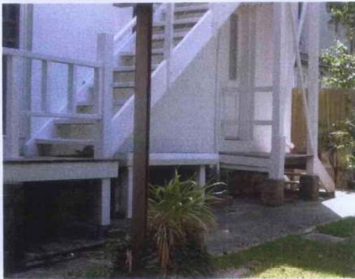
PHOTO 6 Present open stair and landings at rear of dwelling to be removed. New concrete deck to be constructed in this position.
