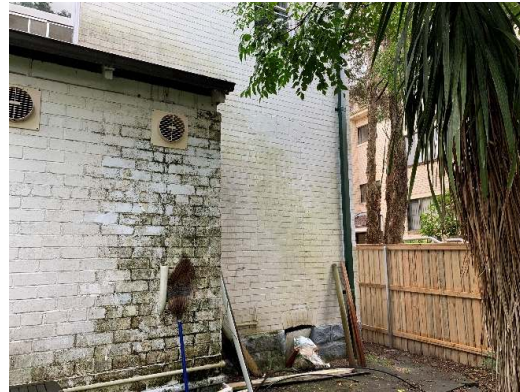
Figure 86. Bricked up opening at ground floor of original dwelling visible in centre of image.
