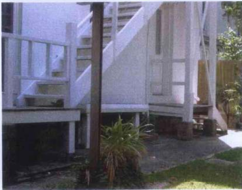
PHOTO 6 Present open stair and landings at rear of dwelling to be removed. New concrete deck to be constructed in this position.
