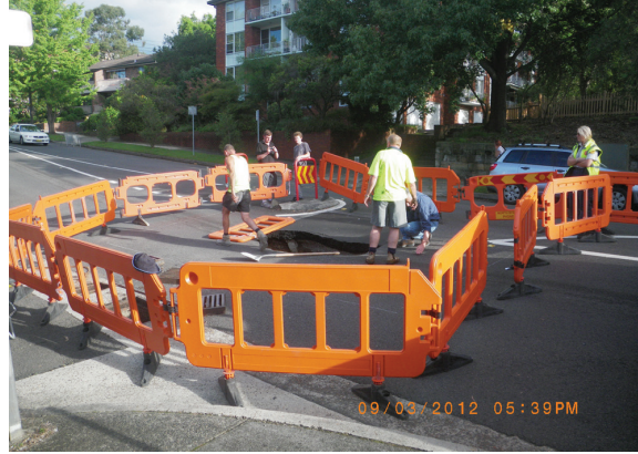
Sink hole in road near defective pipe
