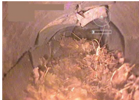
Pipe in very poor condition
