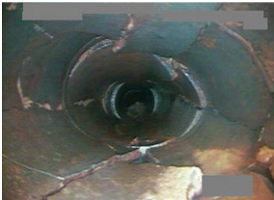
Pipe in very poor condition
