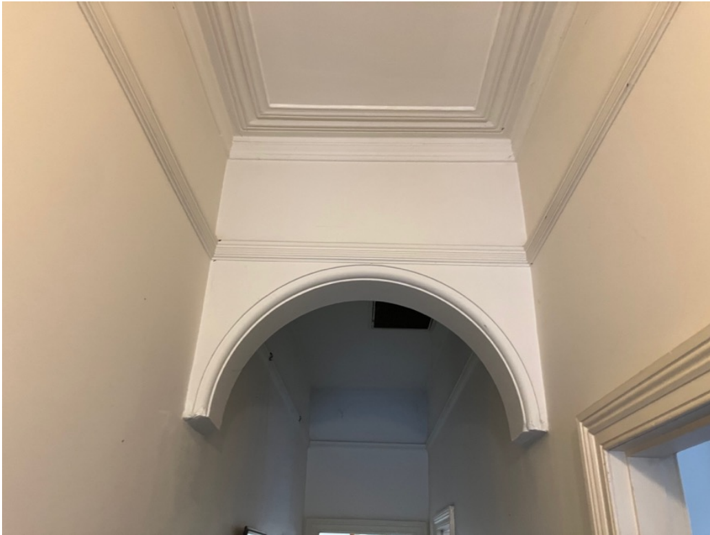
Figure 21: Hallway arch with removed scroll details in No. 27 Bydown Street.
