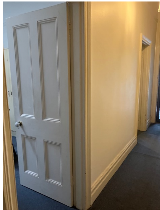
Figure 20: Likely original four panelled door, skirtings, and architraves to main hallway in No. 27 Bydown Street.
