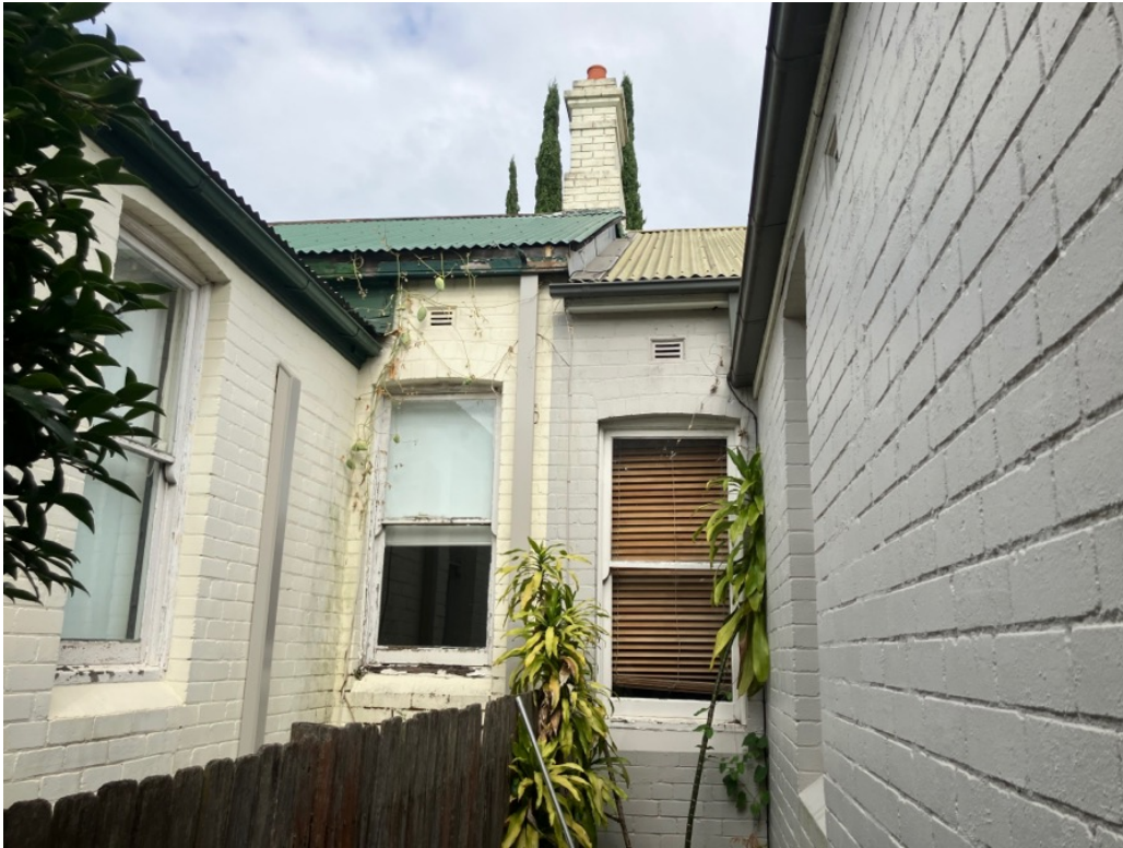
Figure 44: Breezeway between No. 35 and No. 33 Bydown Street with intact form and fenestration
