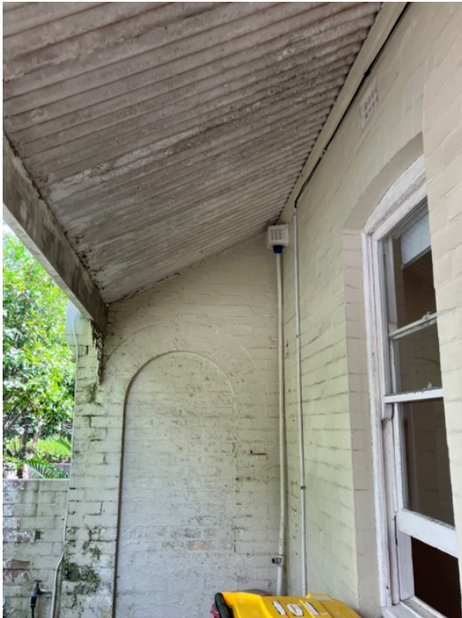
Figure 34: Front entrance verandah of No. 33 Bydown Street showing original form and fenestration.
