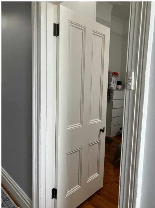
Figure 30: Likely original four panelled door, skirtings, and architraves to main hallway in No.31 Bydown Street and original floors.
