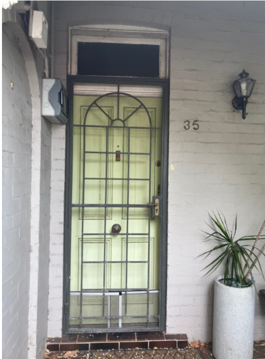
Figure 40: Front door of No. 35 Bydown Street showing original fanlight and modern screen. Original four panel front door with gaps (evident through filtered light) in Figure 42.
