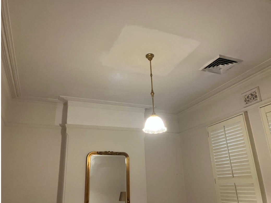
Figure 22: Front room in No. 27 showing cornice and picture rail, vents and removed ceiling rose.
