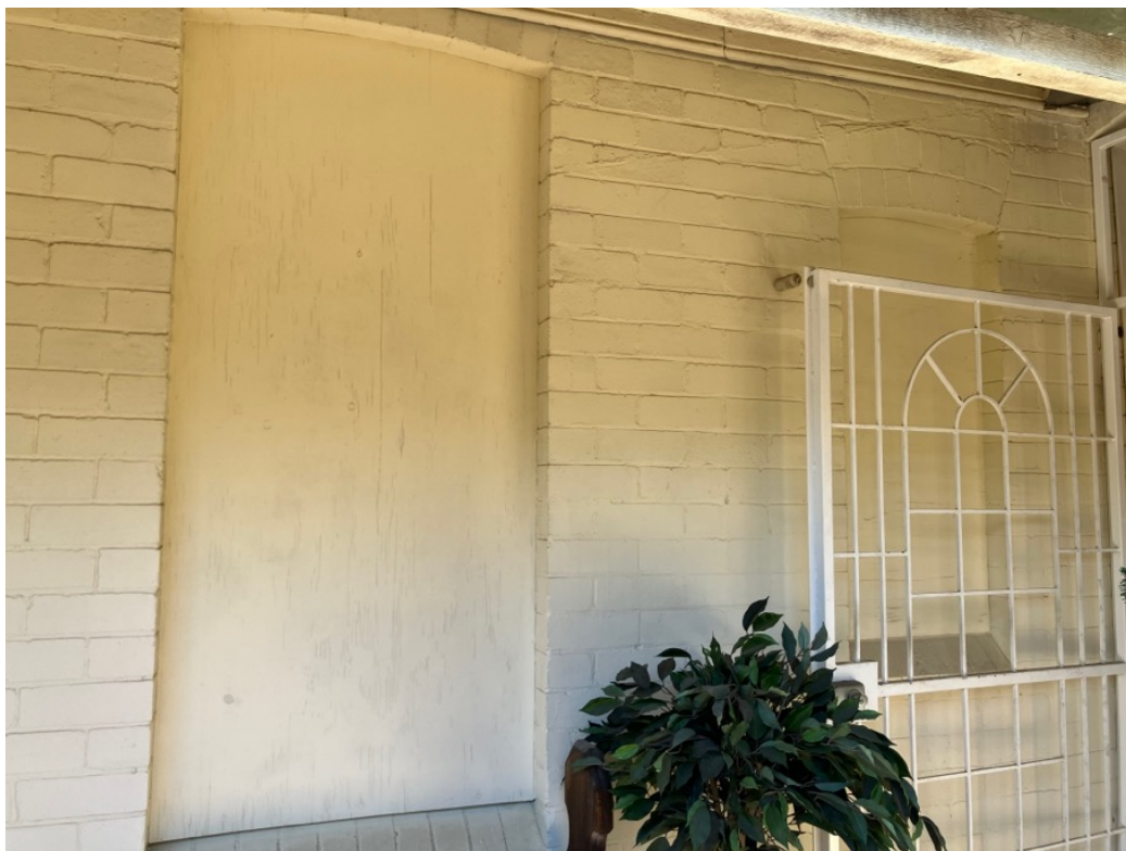
Figure 48: Evidence of original openings at the rear of No. 37 Bydown Street closed off to suit current purpose.
