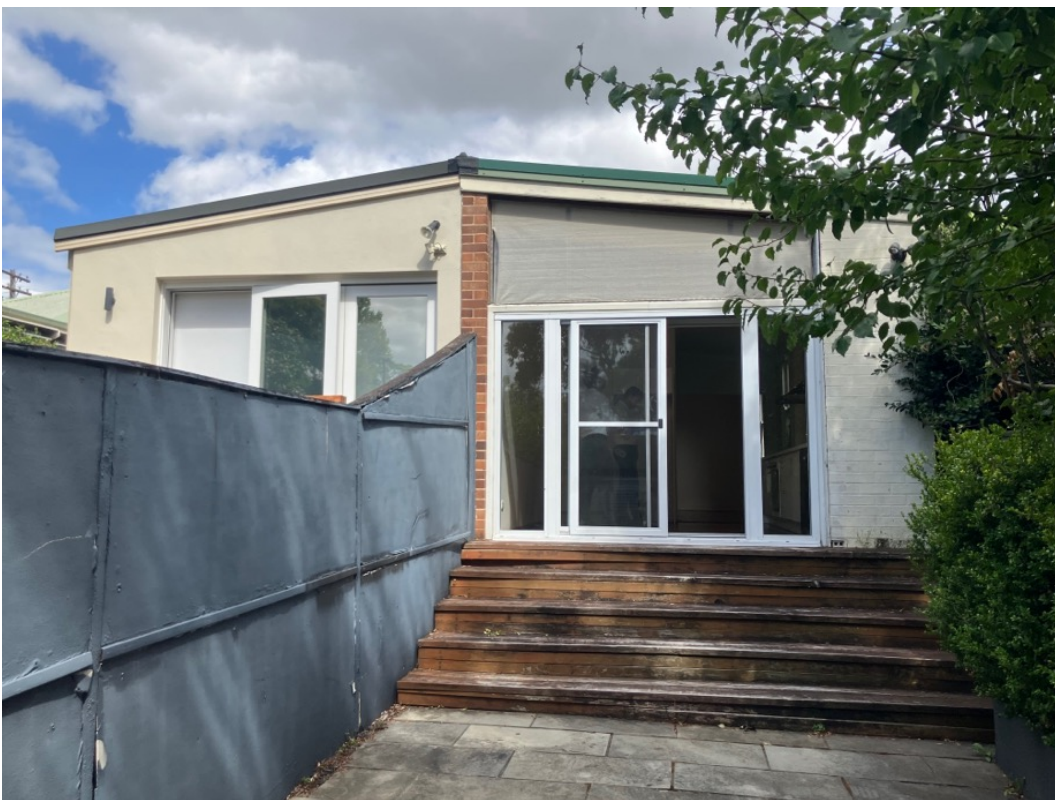
Figure 36: Rear wing of No. 33 Bydown Street, appearing to match the form of its pair at No. 31.
