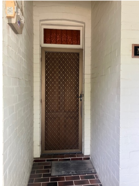
Figure 18: Front door of No. 27 Bydown Street showing original opening and fanlight and modern screen.
