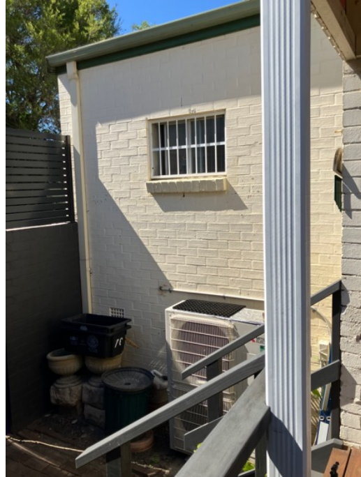
Figure 50: Rear wing of No. 37 Bydown Street, undertaken as part of the 1979 works.
