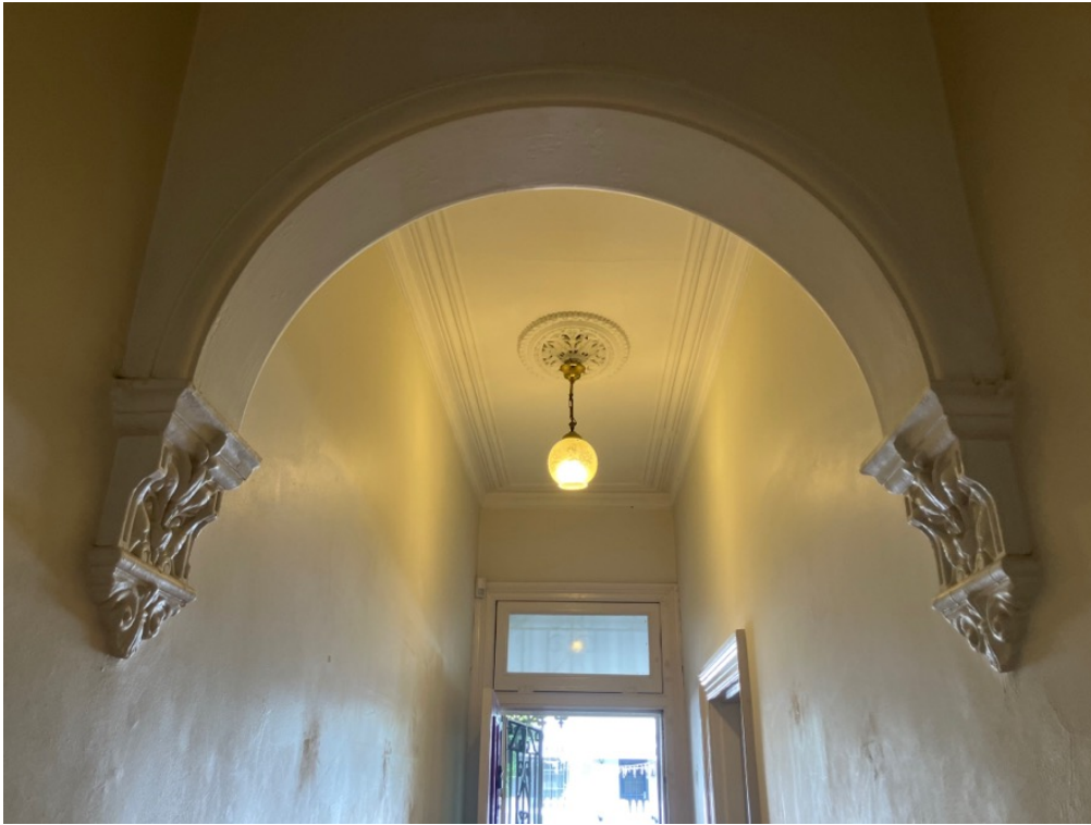
Figure 37: Likely original features of No. 33 including moulded plaster arch, ceiling rose, cornices, architraves, and fanlight over the front door.
