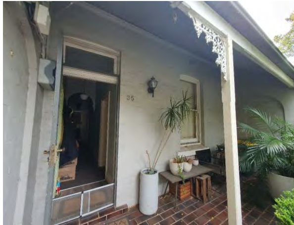
Front elevation – entryway, single timber sash windows, simple timber column, filigree, corrugated sheeting on verandah
