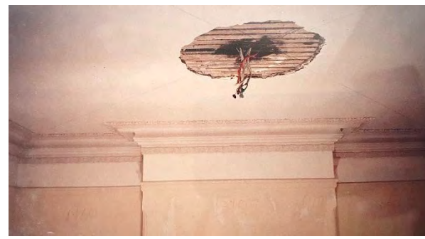
Ceiling of living room during renovations before installation of decorative ceiling rose
