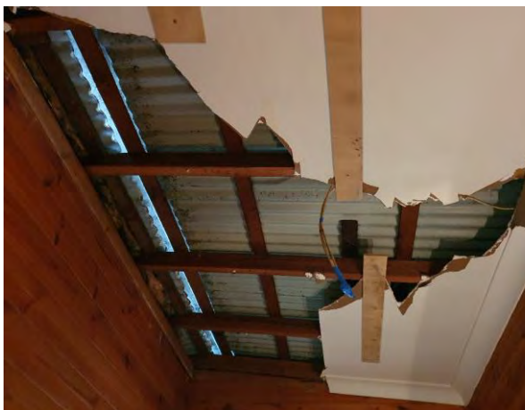
Ceiling and underside of the roof in the bathroom
