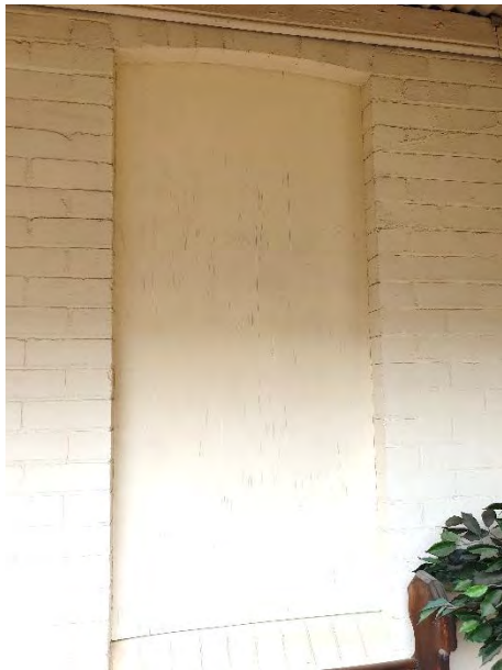
Boarded up window #1
