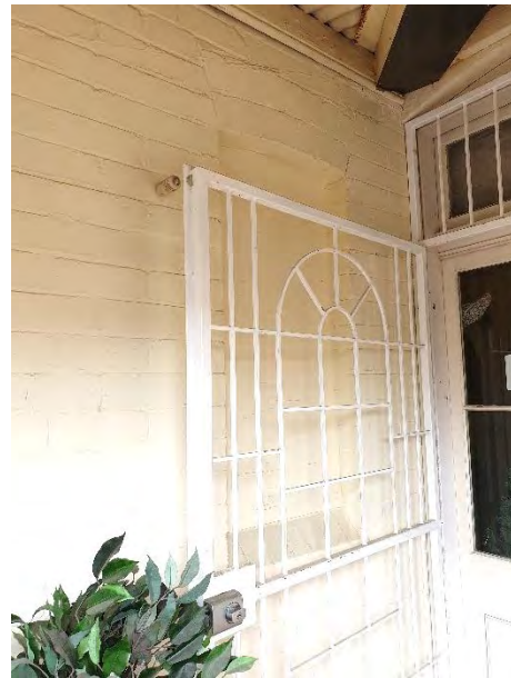
Boarded up window #2
