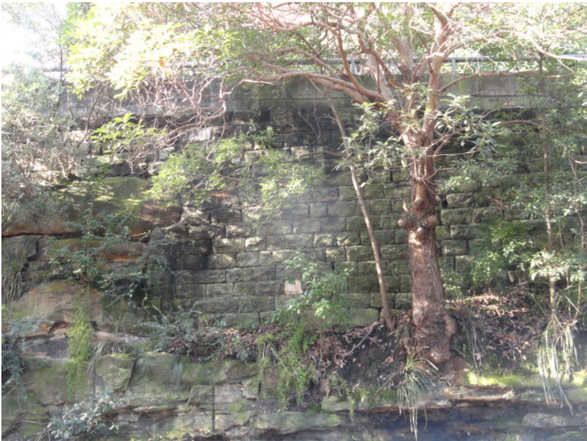
View of the retaining wall from Kurraba Road showing the road barrier on top of the sandstone retaining wall founded on sandstone
