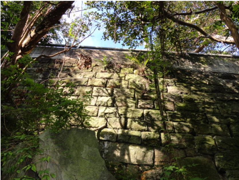
Western sector: View of bulging section with opening of perpends
