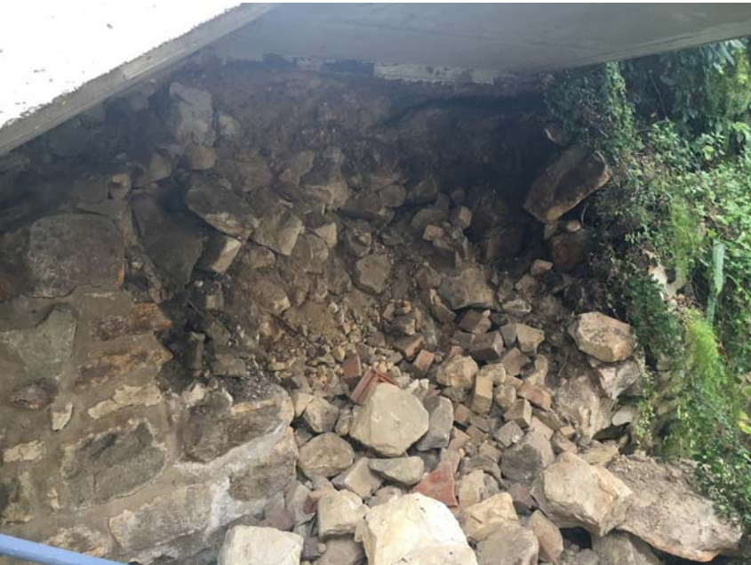
Collapsed wall at 102 Macpherson St
