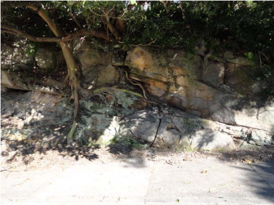
Fig tree with roots “wedging” into rock joints and loose rocks on embankment requiring treatment.
