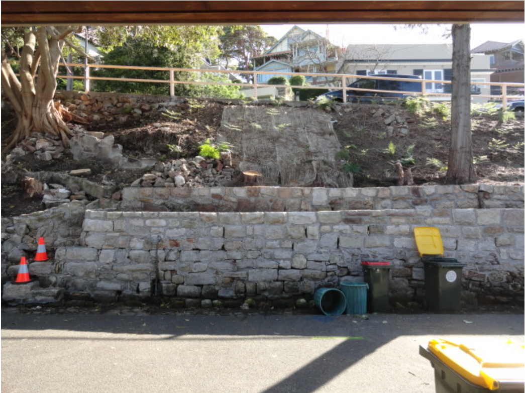
View of embankment adjacent to property no. 42. Note the partial collapsed of the wall just below the timber fencing.
