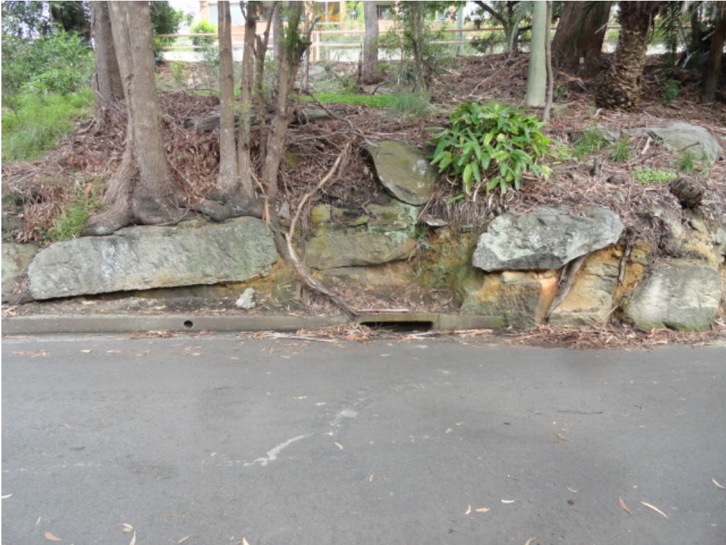
Additional erosion of the embankment destabilizing the rock outcrop
