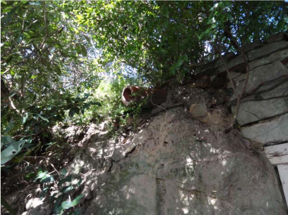
View of unstable earth embankment and disconnected stormwater line on east side of garage entry to property no. 66
