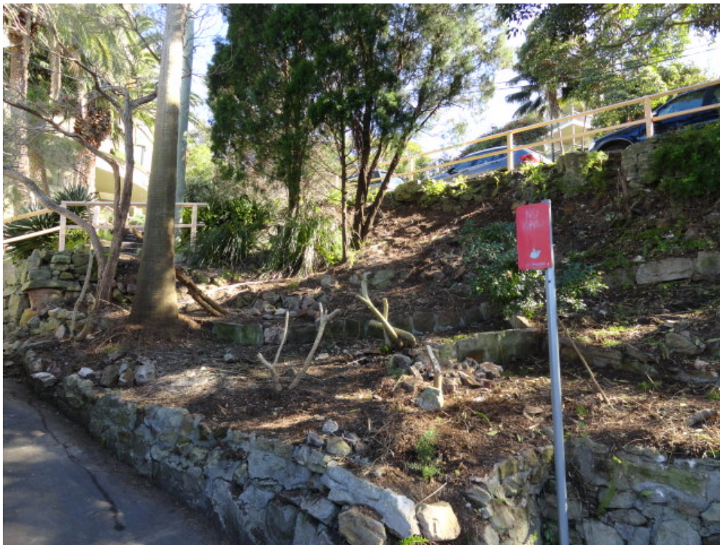
View of embankment adjacent to property no. 44. Note very poor condition of stone retaining wall at base.
