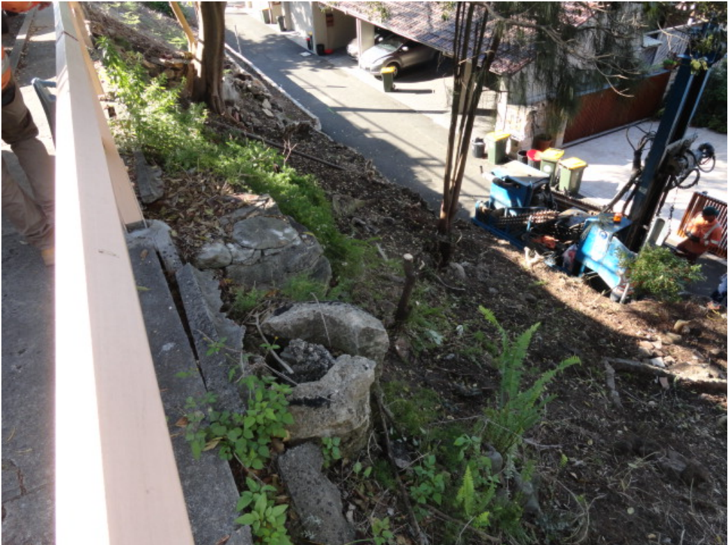
View of western edge of footpath opposite property no. 42 from the high side of Milsons Rd. Note settlement of fill and movement of stone walls.
