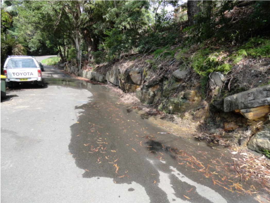
View of the eroded embankment
