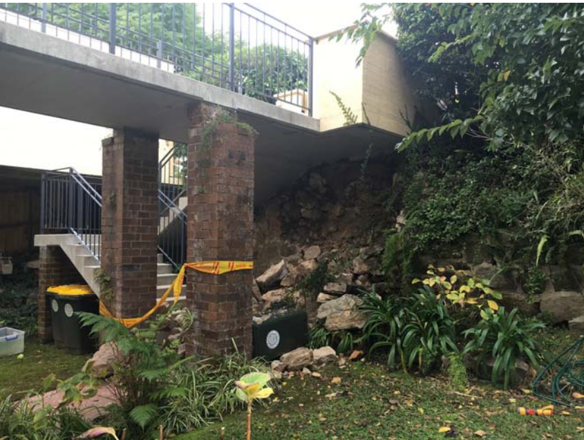
Collapsed wall under footbridge
