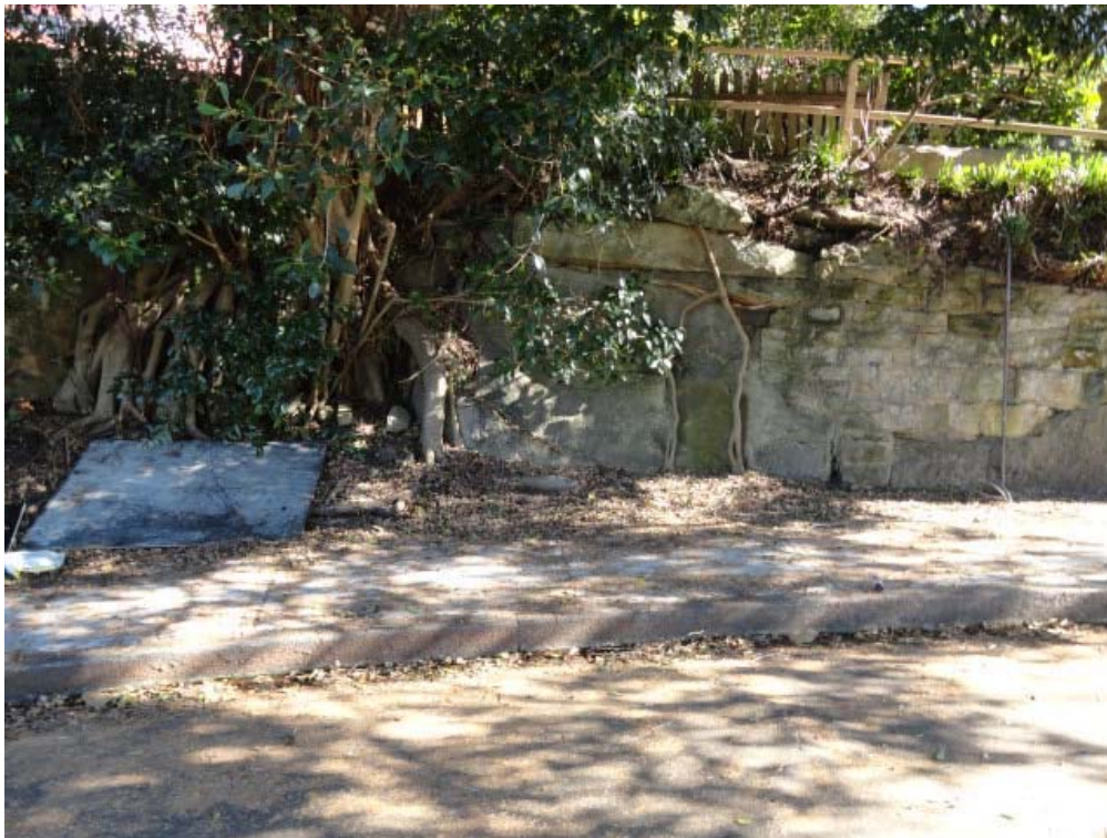
Footpath above embankment shows signs of lifting outside entry to no. 66
