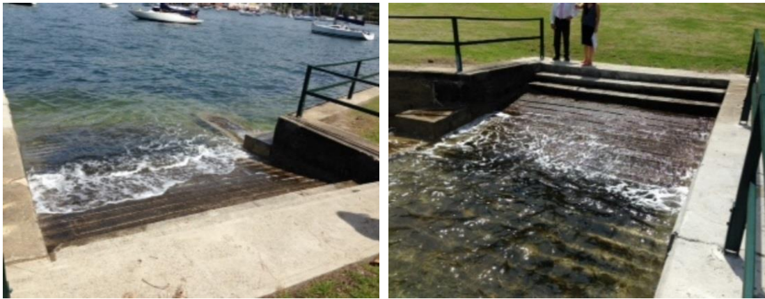
Existing launching ramp for small water craft at Kurraba Reserve, Neutral Bay
