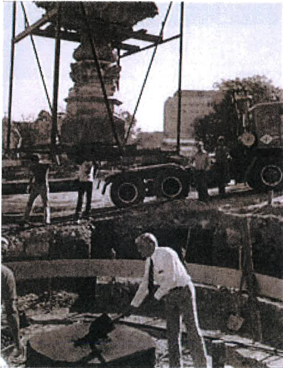
Mayor Ted Mack shovels concrete onto base ready for positioning of the Queen Victoria Jubilee Fountain in the Civic Centre, North May 1982.
