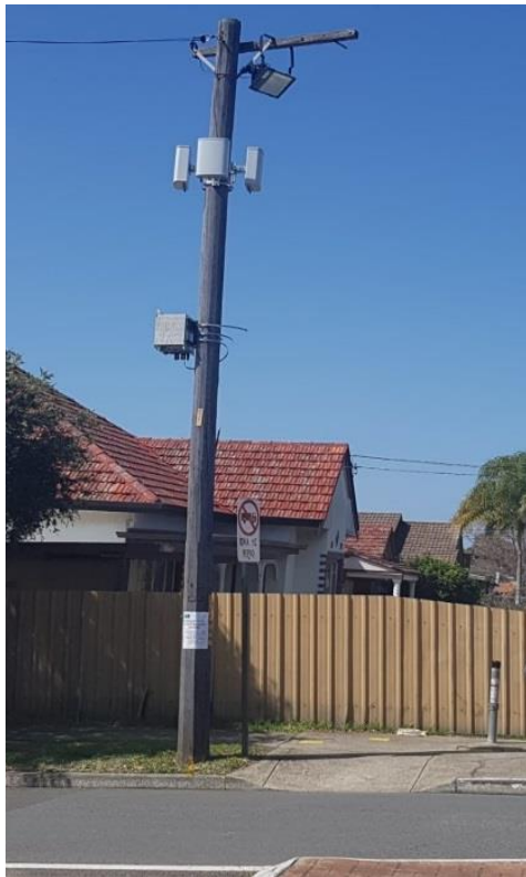
Photo 1 – typical image of micro cell telecommunication facility recently installed on a power pole in the Canterbury Bankstown area
