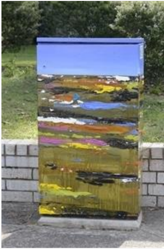
Box 22. Ben Boyd Rd cnr Yeo St, Neutral Bay
